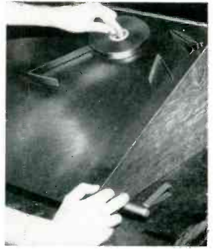
Rewinding tape into flat wad that is easily shoved under cable. Completed wad is at upper right on steel table, with fishpaper core under it
