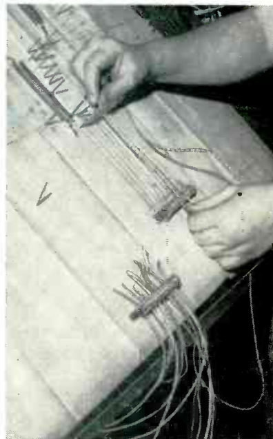
How pre-stretched coil springs are used for holding wire ends on cable harness board at DuMont plant
